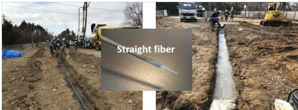
Fig. 4. (left) Distributed fibre optic Strain Sensing (DSS) cable installed in a trench; (right) DSS cable covered with cement [1].
